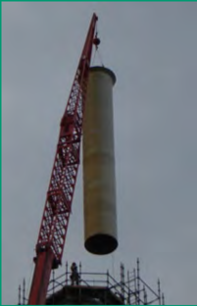
Stack liner, 6' diameter x 40' section of 200' stack
