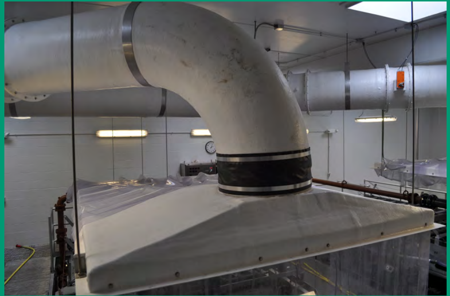
FRP Odor Control Hoods and Ducting
