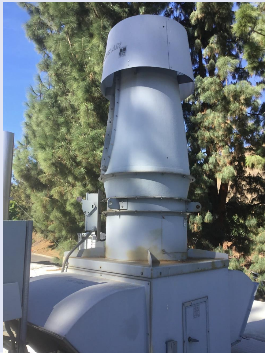
Before – (HCl application – Fan destroyed Painted Steel Product )
