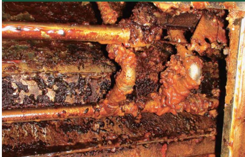
Hood without JIMCO UV-C Technology - not cleaned for 6 months
