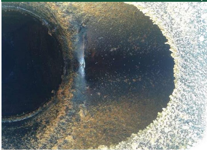
Fryer Duct without JIMCO UV-C Technology - not cleaned for 12 months :
