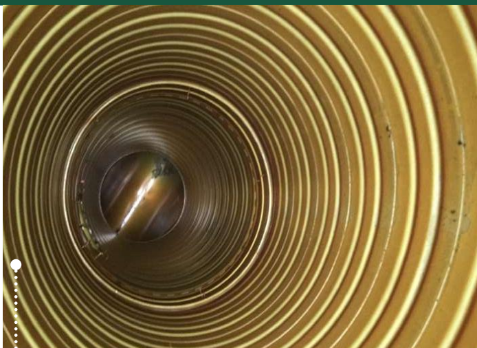
Fryer Duct with JIMCO UV-C Technology - not cleaned for 60 months
