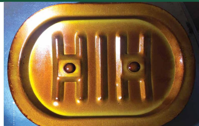
Inspection Hatch with JIMCO UV-C Technology - not cleaned for 60 months
