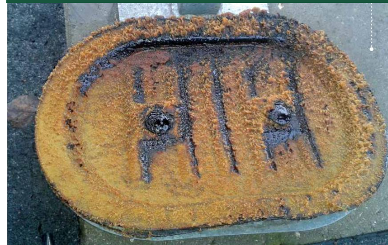
Inspection Hatch without JIMCO UV-C Technology - not cleaned for 12 months
